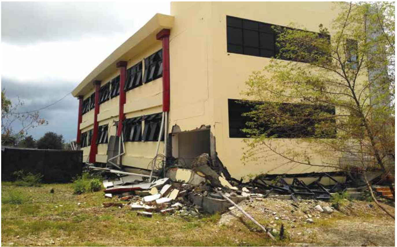
A building collapsed due to the earthquake in Palu, September 2018
