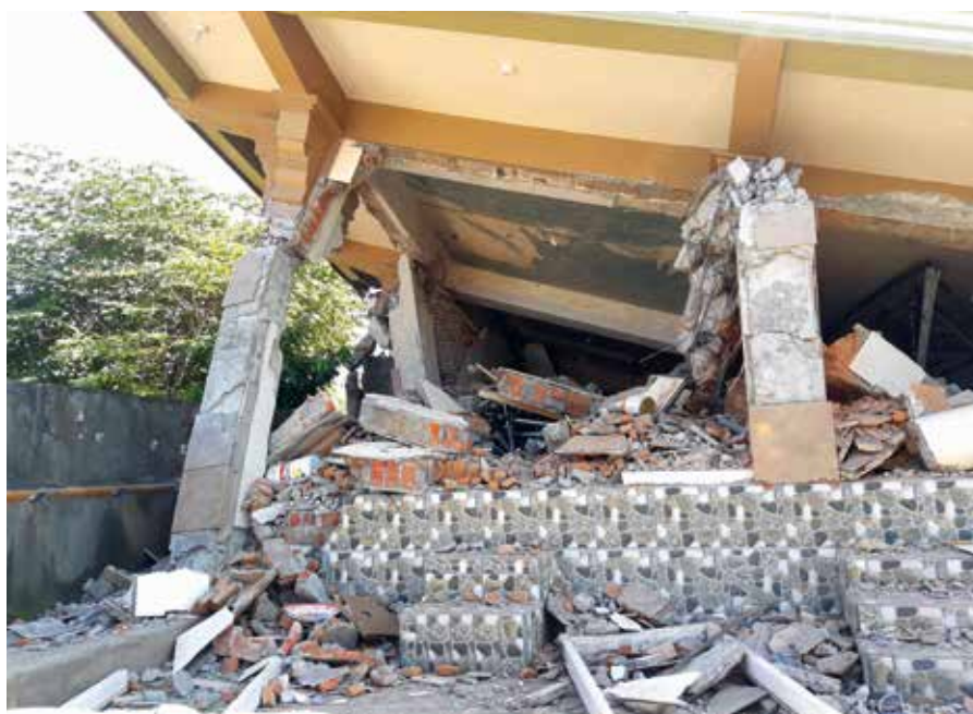
Impact of severe damage during the Lombok earthquake in 2018
